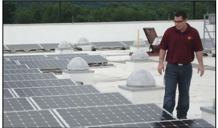
Construction Intern/Clerk of Work Samuel Roit inspects a Solar Array recently installed by Goldbelt on the NETL Daycare Center in Morgantown, West Virginia.
